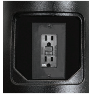
GFI IB 15 amp duplex GFCI receptacle installed in pole base, includes mouse hole on door for wire access
